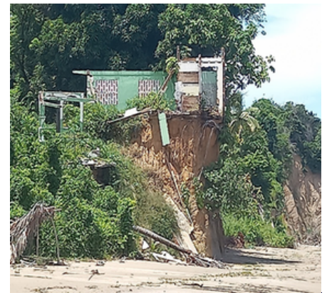
House on edge affected by land slippage
